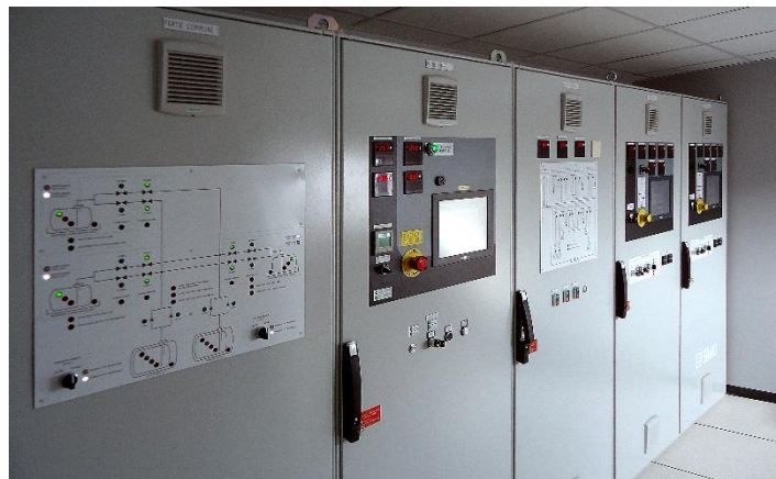
Pic. 2: Electrical cabinets of the gensets
